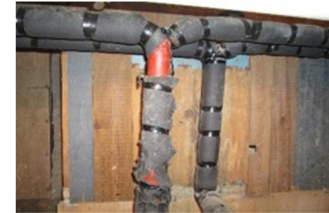
Poor quality of technical insulation
