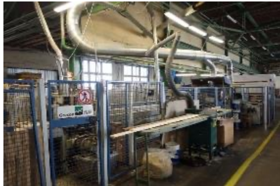
Compressed air systems
