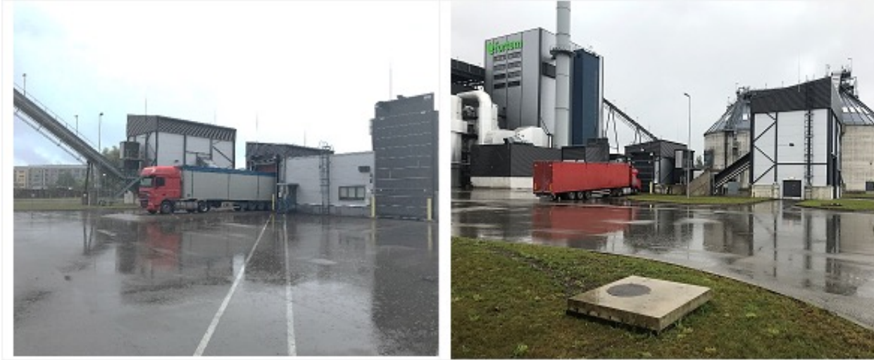
Fuel reception area
