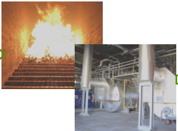
2012 new 7 MW wood chips boiler and new gas boilers
